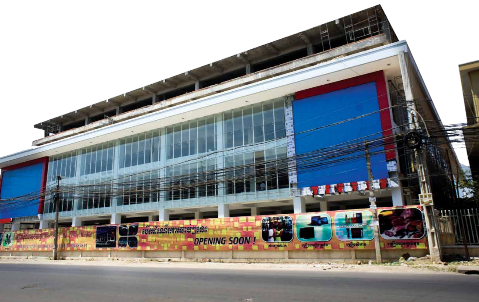
📍 Uplift in Area: New Stung Meanchey market is under construction. The new market is expected to change the life style of citizen in region. (Photography by Meas Proeksa)
