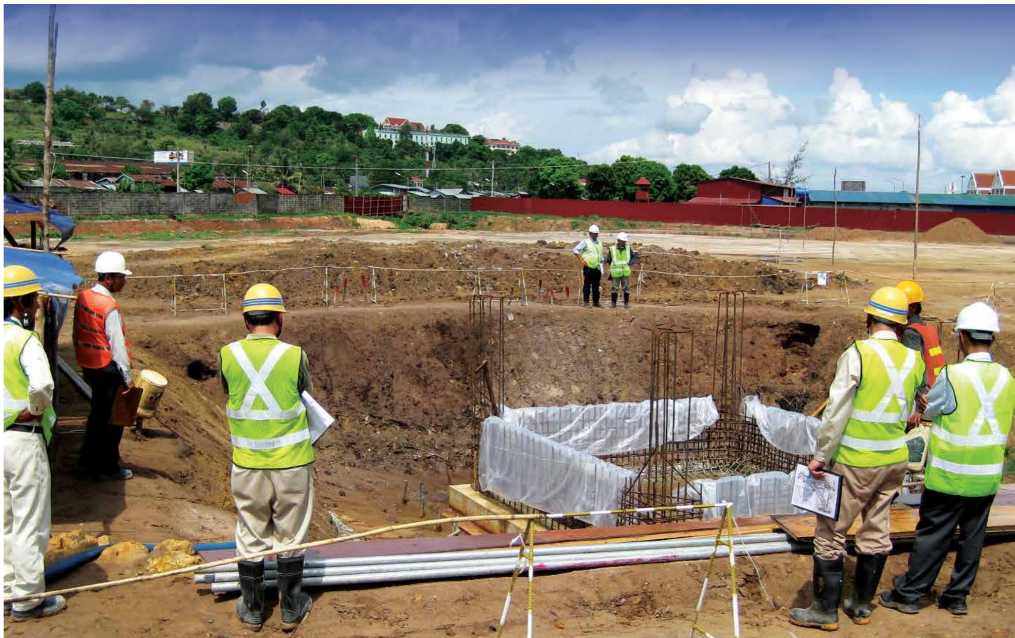
Consultant's inspection rebar before concrete casting work at Sihanoukville Port Special Economics Zone
