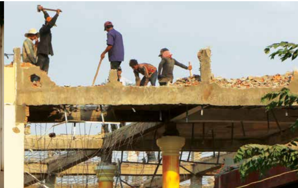
Unsafe working condition at a building demolition work in Phnom Penh
