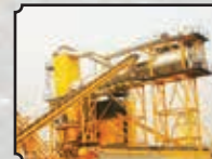
HRC - Hot Recycling Plant
