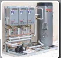
Centralized Gas Hot Water System
