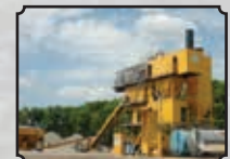
CSD - Containerized Plant
