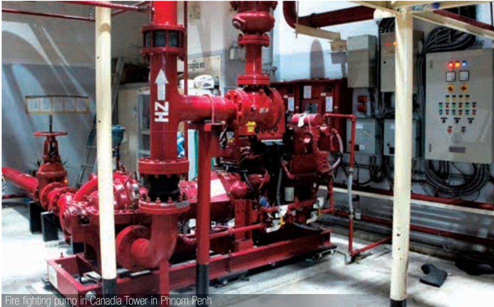
Fire fighting pump in Canadia Tower in Phnom Penh
