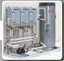
Centralized Gas Hot Water System
