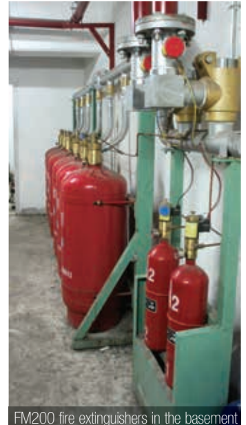
FM200 fire extinguishers in the basement
