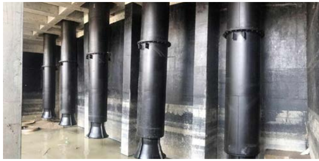
▼ Five more water draining machines installed at Boeung Trabek station to cope with flooding
